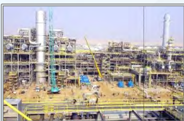
Nghi Son Refinery Thanh Hoa
