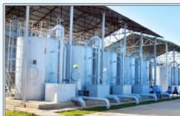
Ngoc Tuan Water Plant Hung Yen
