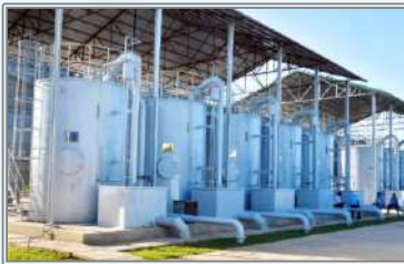
Ngoc Tuan Water Plant Hung Yen
